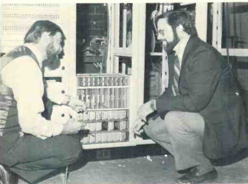
The WWAC plant was done on a turnkey basis with much of the assembly done on the erection floor at Peirce-Phelps' Philadelphia plant. Peirce-Phelps' chief engineer, Donald B. Leith goes over some of WWAC's rack-mounted equipment with staff engineer James Ridenour (right)
